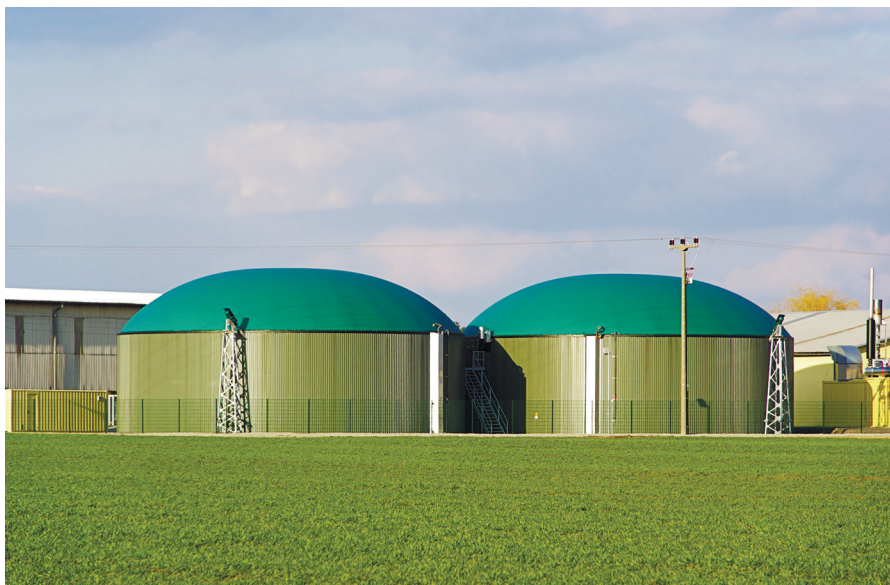
Figure 3-23: Typical farm-based vertical digester system
